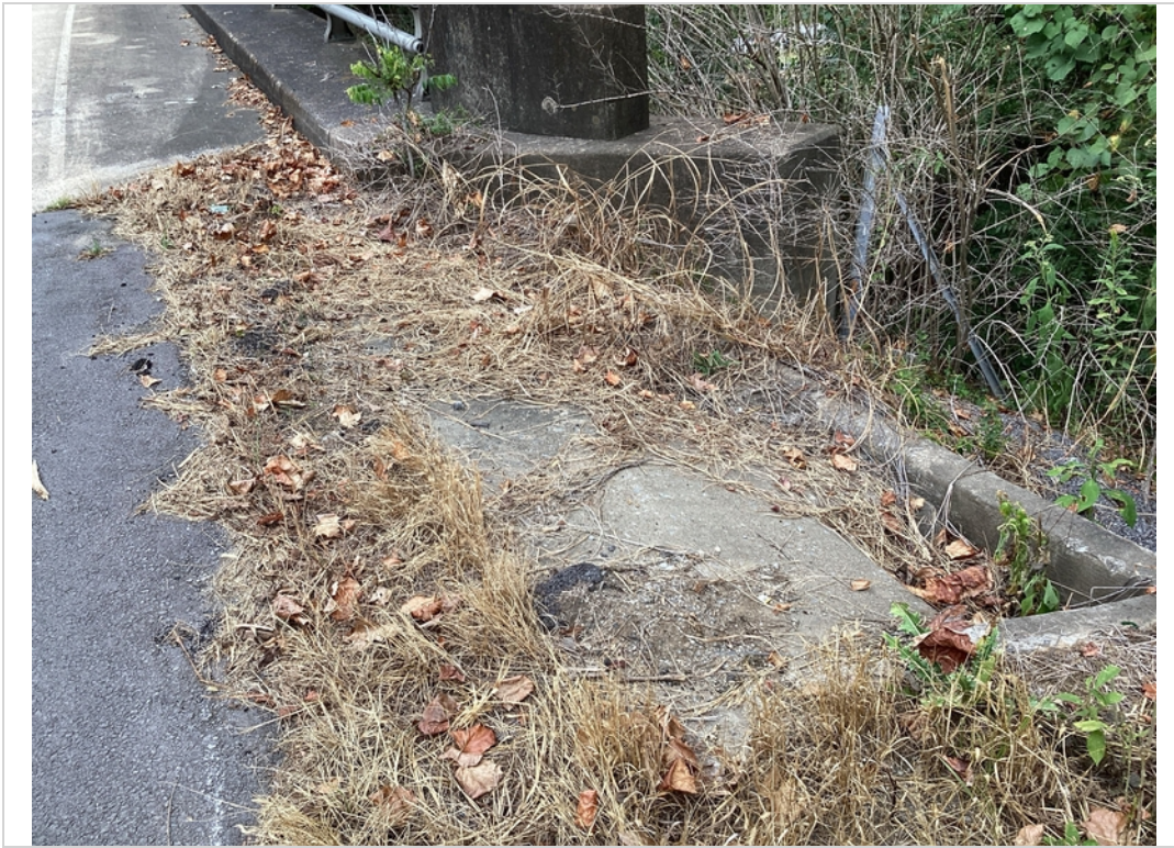
Approach 2 left drain - debris and plugged
