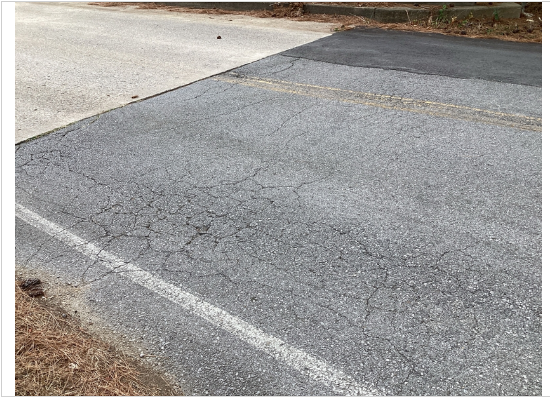
Approach 1 wearing surface - patch, cracks to 1/8"
