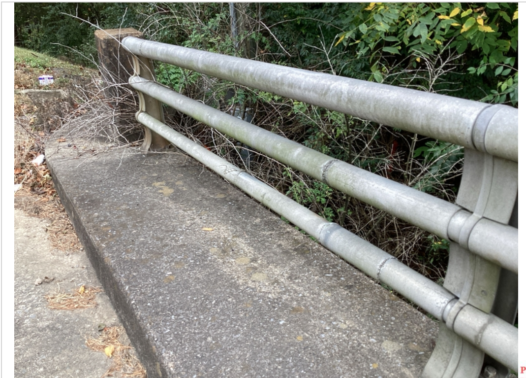
Deck 4 right bridge rail - loose
