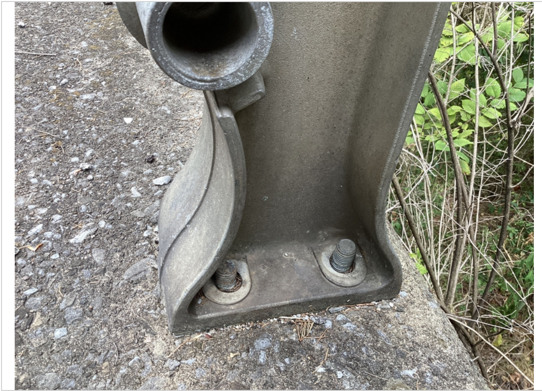
Deck 4 left bridge rail post back - missing nuts (also missing one on front)
