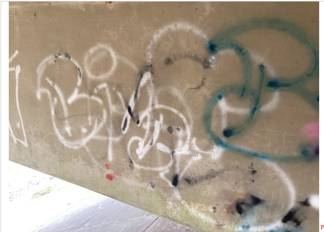
Beam A - abutment 1 - graffiti
