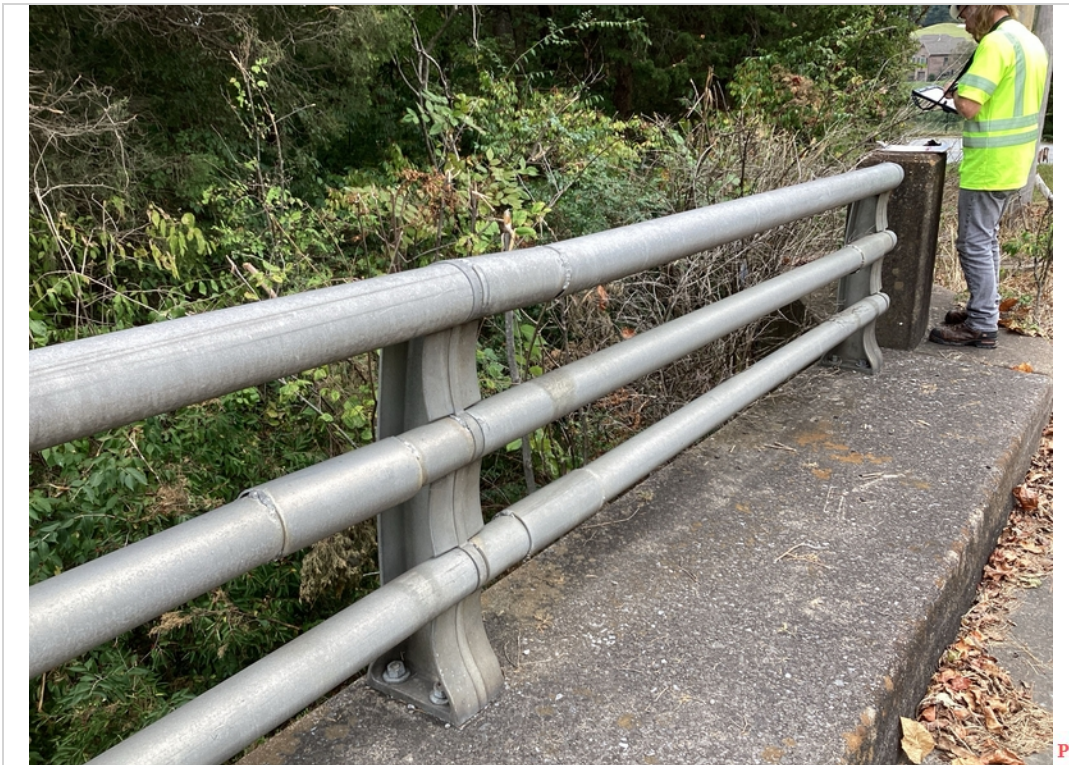
Deck 4 left bridge rail - loose
