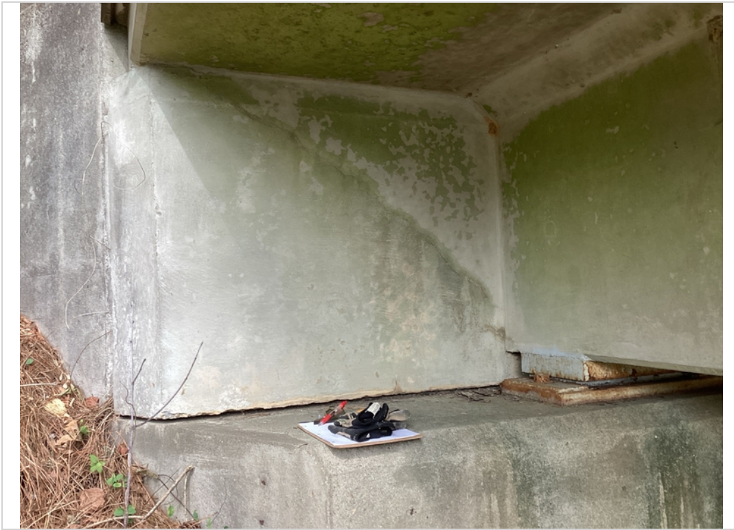
Backwall abutment 1 - Hairline cracks
