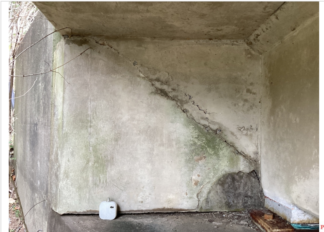
Abutment 2 left Backwall at beam A left - 1/16"
