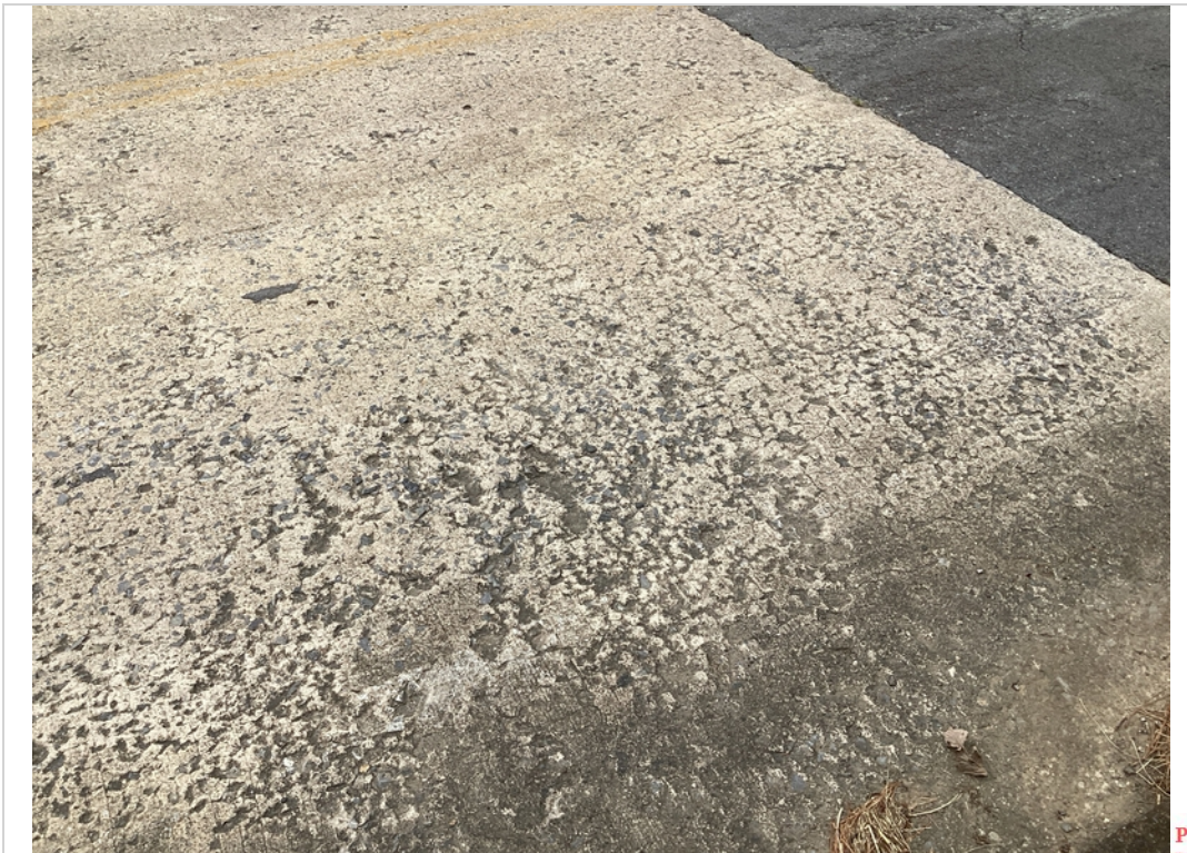
Deck 4 right at approach 2 - area moderate scale
