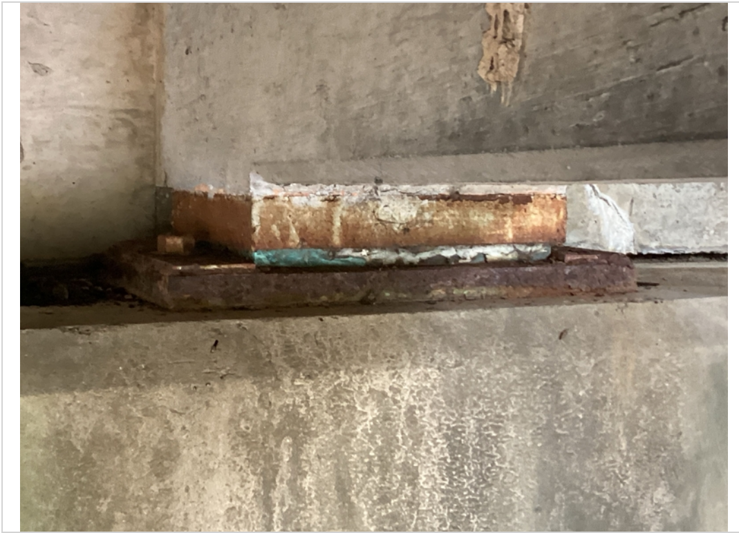
Abutment 2 - Bearings A & D - moderate corrosion
