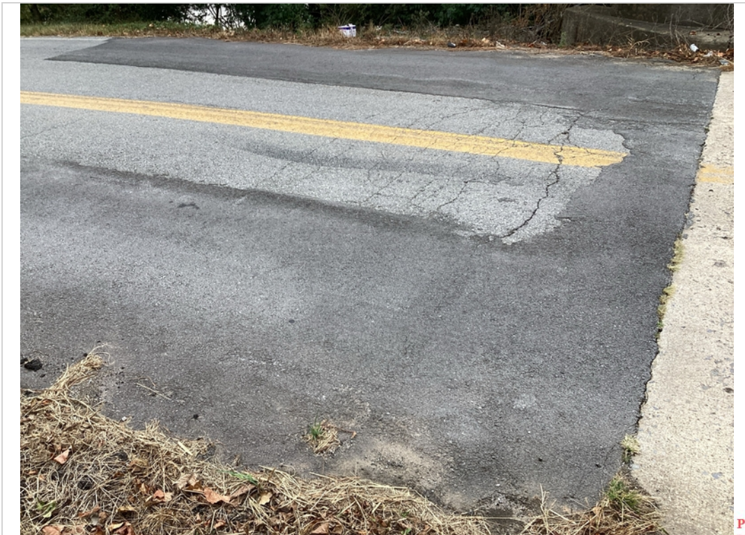
Approach 1 wearing surface - patches, cracks to 1/4"
