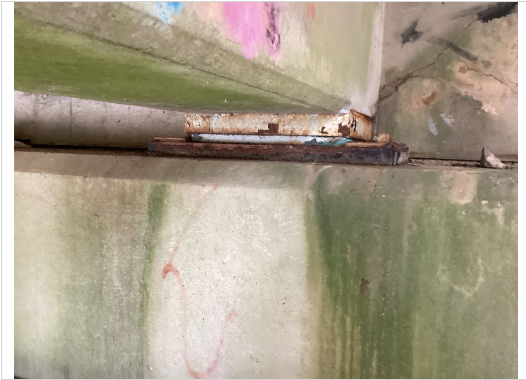
Abutment 1 - Bearing A - moderate corrosion
