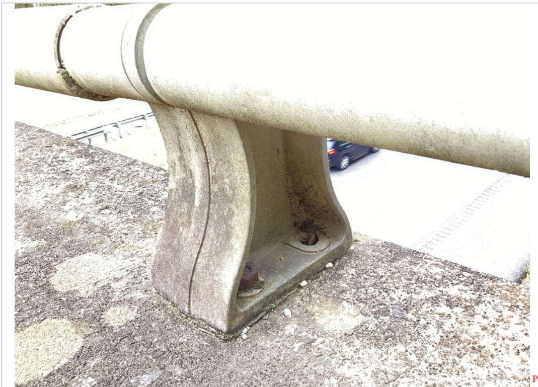
Deck 2 right rail post front- missing bolt ( also missing nut on back side)
