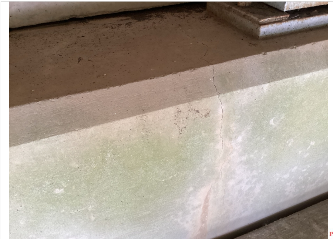
Abutment cap 1 - Hairline cracks (Typical abutment 2)
