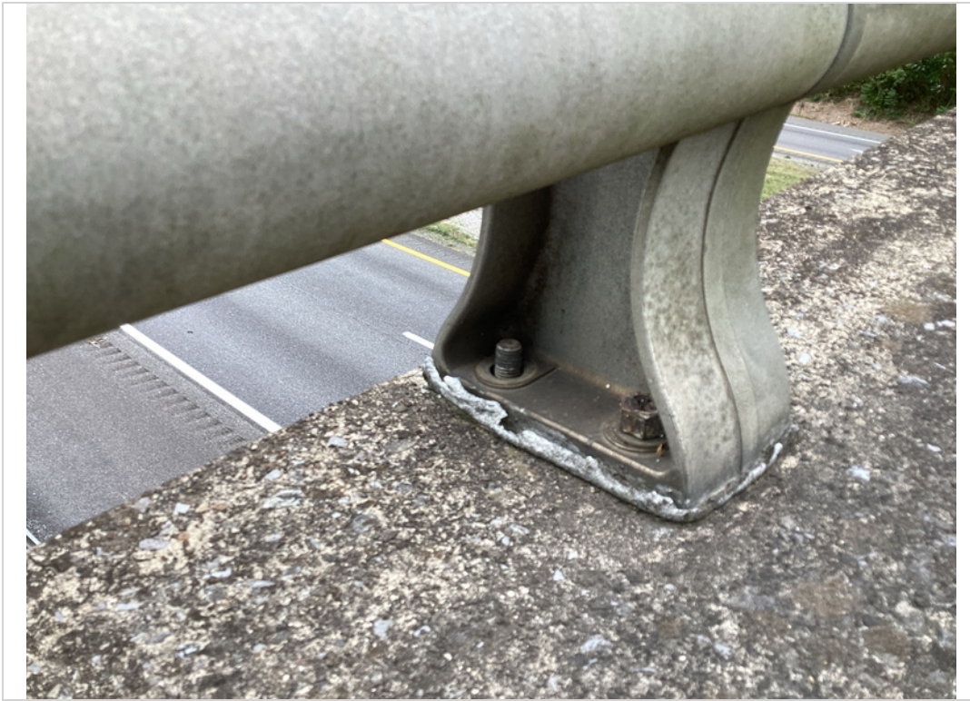
Deck 3 right rail post - missing nut
