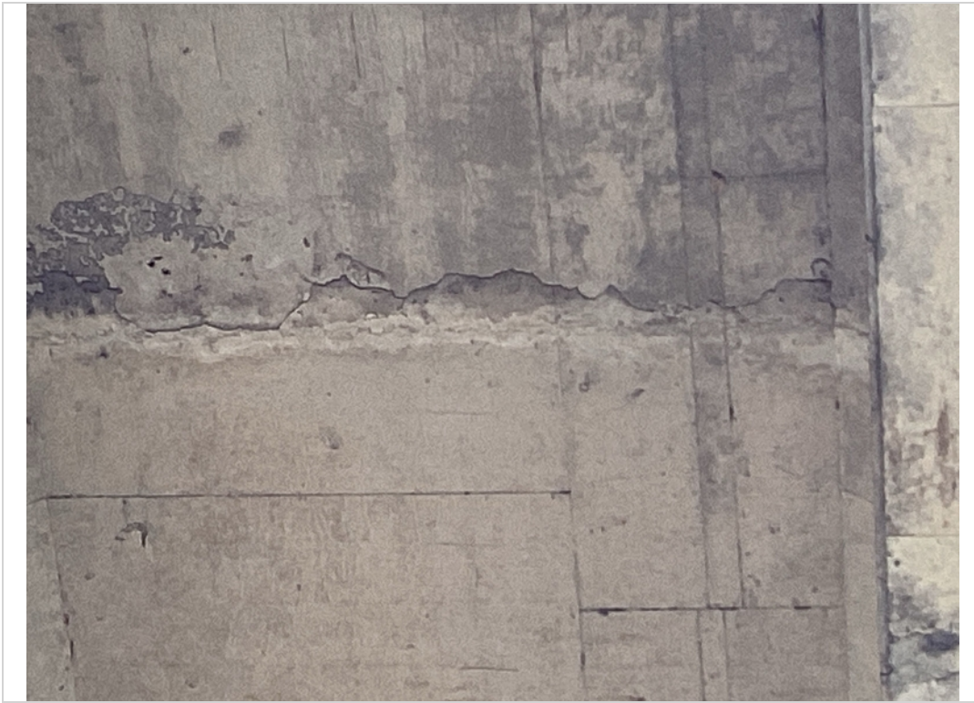
Span 1 bottom deck between beams A & B - Cracking up to 1/8" with leaching at the construction joints
