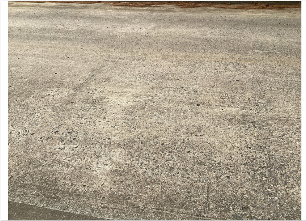
Deck 1 wearing surface - hairline map cracks, light scale, few aggregate voids
