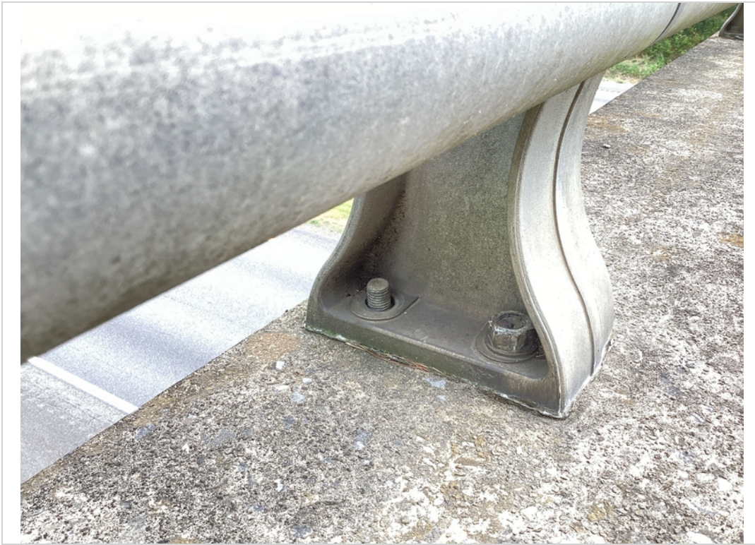
Deck 2 left rail post front- missing nut (also missing nut on back side)
