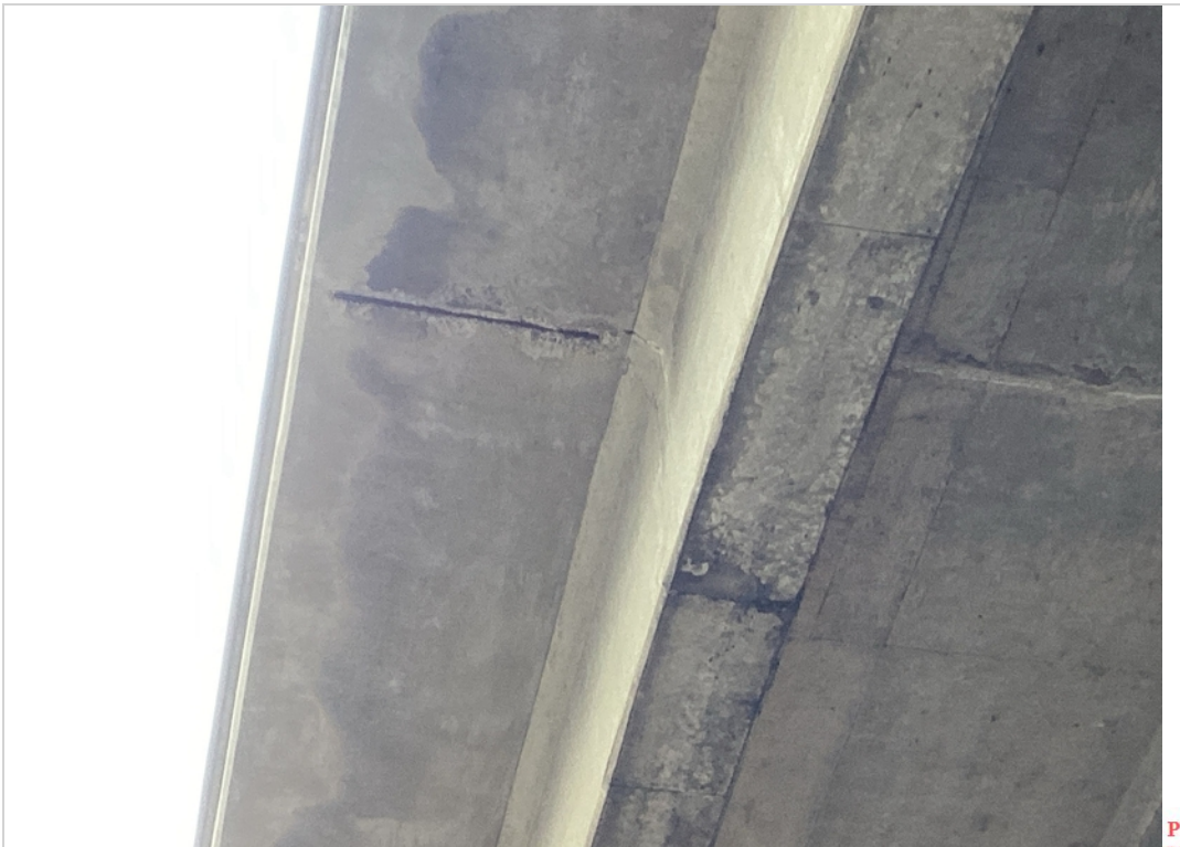
Span 2 left overhang - Popout and Hairline cracks with leaching
