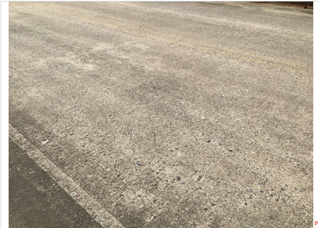
Deck 2 wearing surface - hairline to 1/16" map cracks, light scale, few aggregate voids
