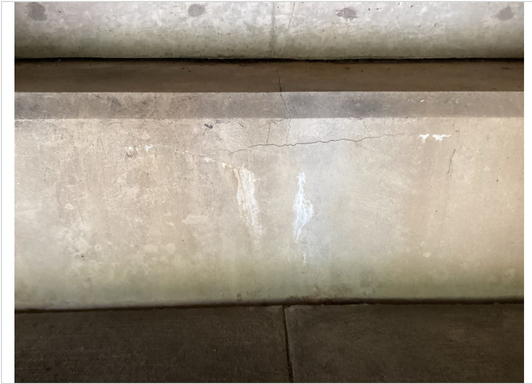
Abutment cap 2 - Cracks up to 1/16" & hairline cracks w/ leaching
