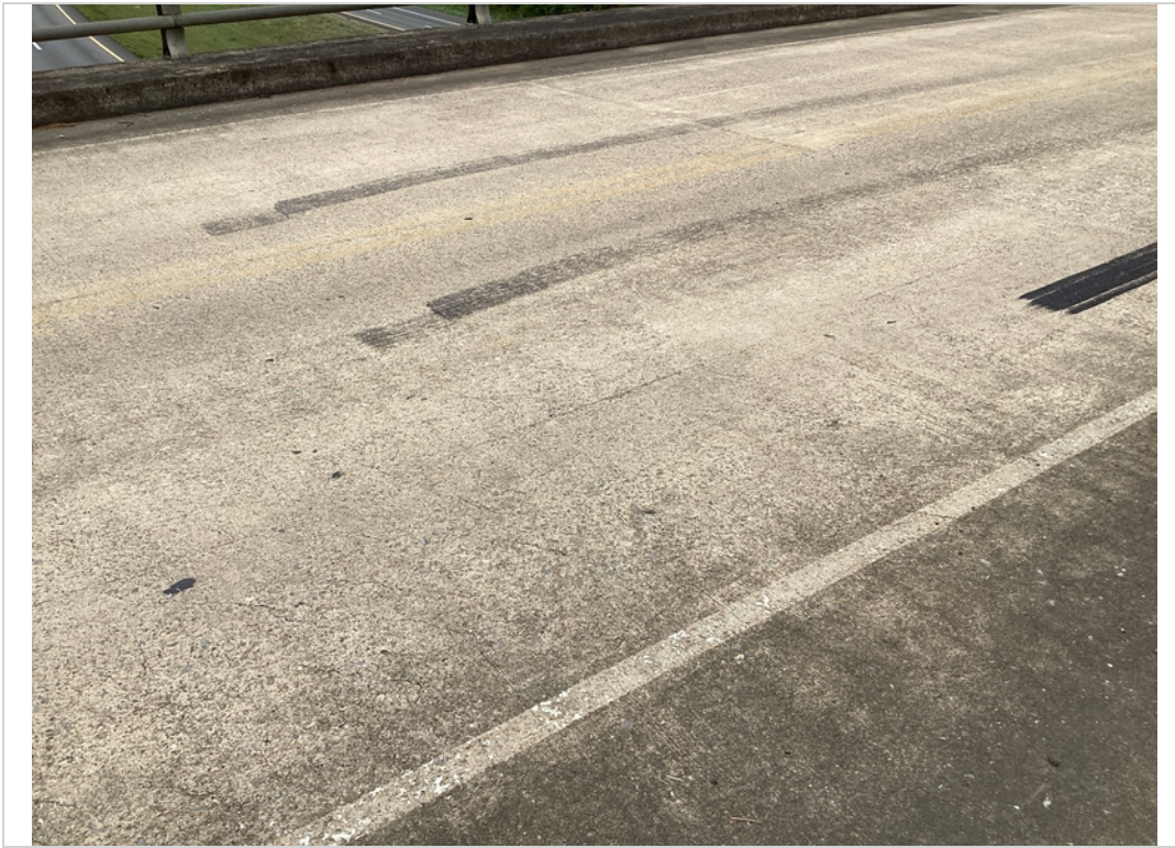
Deck 3 wearing surface - hairline to 1/16" map cracks, light scale, tire marks
