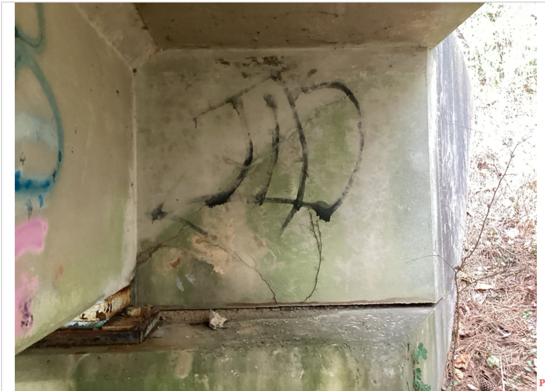
Abutment 1 back wall - Cracking up to 1/8"
