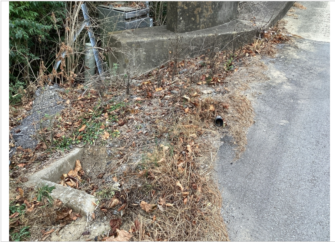
Approach 2 right drain - debris and plugged
