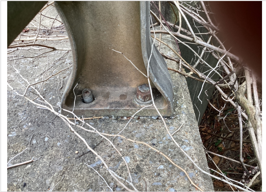
Deck 4 right bridge rail post - loose, missing nut
